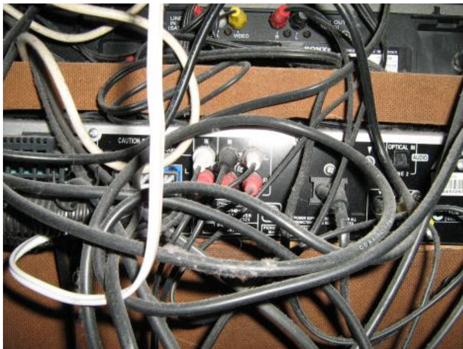
Figure 3: Complexity in cabling
